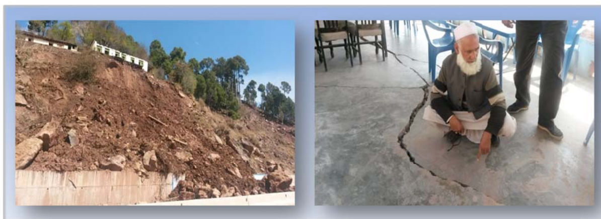
Figure 1: Landslide along the road from Islamabad to Muzaffarabad (left); on the right: cracks in the ground slab of a house immediately placed below the road level (Source: D. BALZER, taken 2014).
