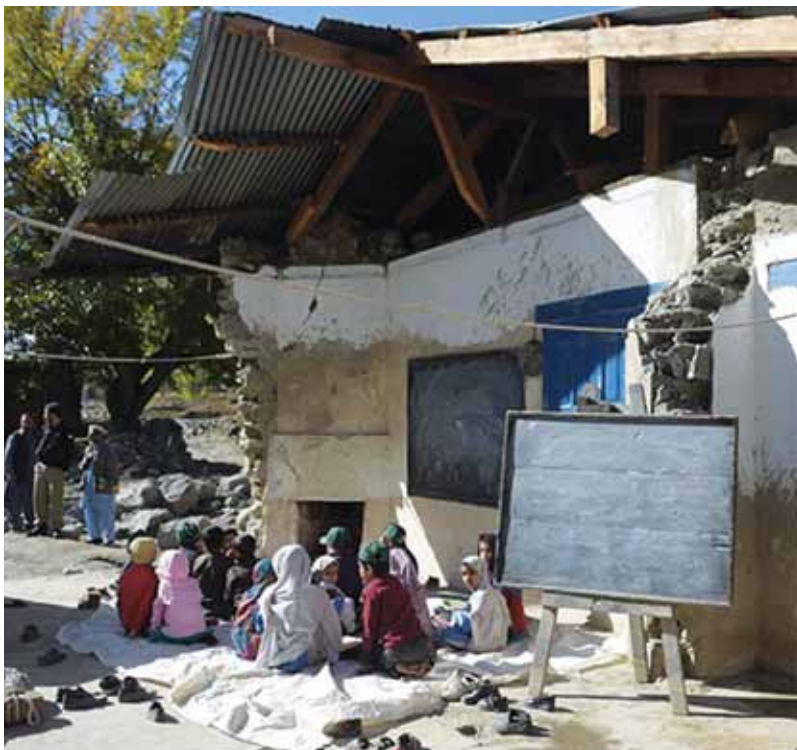
Earthquake affected school at Brun Chitral
