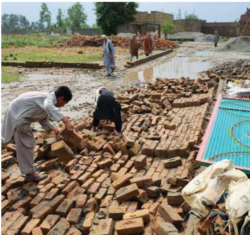
Damages at Baila Niko Khan Peshawar
