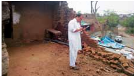
Damages Need Assessment activity in affected area of Peshawar
